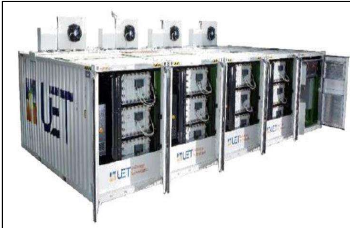
Figure 10: Flow Batteries - Vanadium Redox Battery
