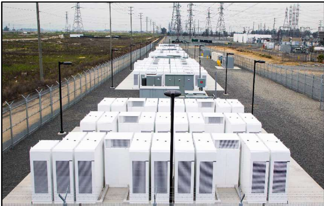
Figure 9: Solid State Batteries (Lithium-ion)
